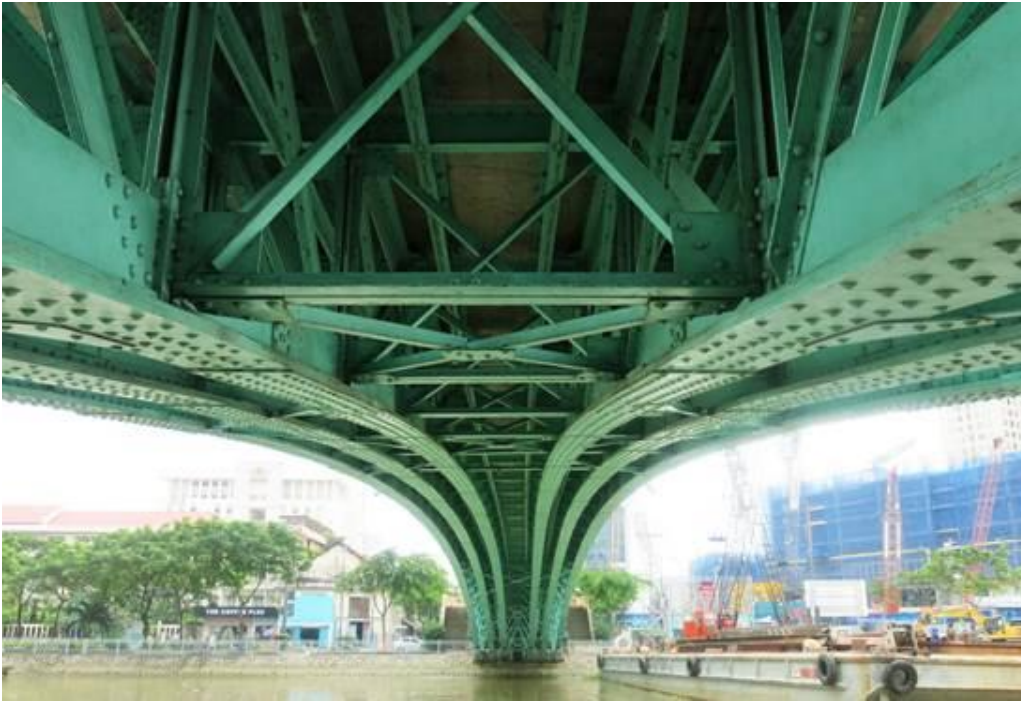
The 'Rainbow Bridge' (Pont des Messageries Maritimes or Pont de Khanh-Hoi), Ho Chi Minh City by les Établissements Eiffel, 1882, underside: Miles Lewis.
