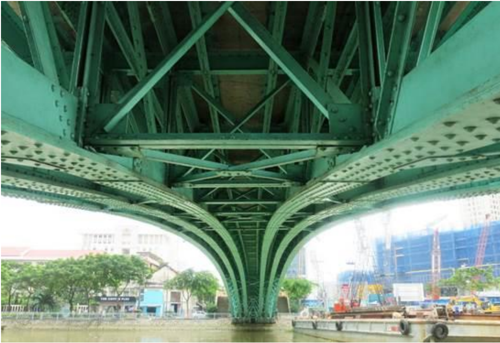
The 'Rainbow Bridge' (Pont des Messageries Maritimes or Pont de Khanh-Hoi), Ho Chi Minh City by les Établissements Eiffel, 1882, underside: Miles Lewis.
